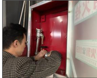
Photo of fire safety equipment fire hydrant.JPG
