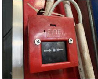
Photo of fire safety equipment fire alarm.JPG
