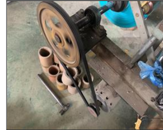
Photo of non-conformity NC - missing safety guard.JPG
