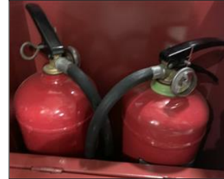
Photo of fire safety equipment fire extinguisher.JPG
