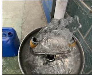
Photo of the inside of the main production hall eye wash facility.JPG
